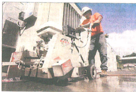
Ed Villarreal of Sonoma Engineering cuts asphalt Friday in preparation for a new $3 million emergency room being erected at the hospital.
